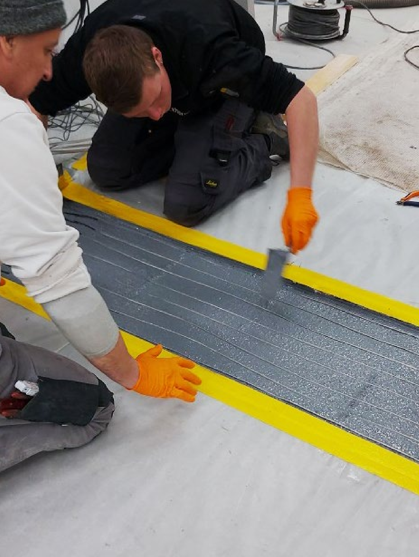
Installation of a special Tensa®POLYFLEX® plug-type expansion joint beneath the rolling door of a frozen storage room, with heating elements placed between layers of the joint's elastic PU material to prevent the door from becoming frozen closed.
