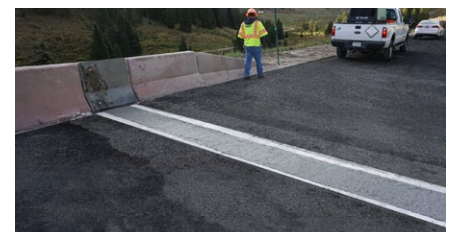
The completed flexible plug expansion joint high in the Rocky Mountains of Colorado
