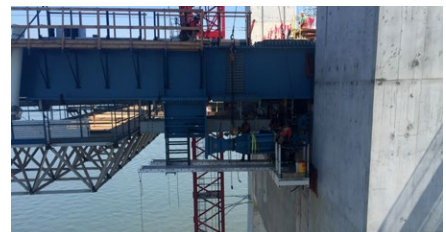
Installed shock transmission unit
