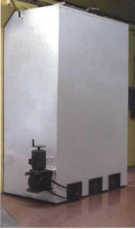
Above: EPD Concrete-Filled Shielding Door; rolls into place on a track at the AMF Baird X-ray facility, Baton Rouge, Louisiana
