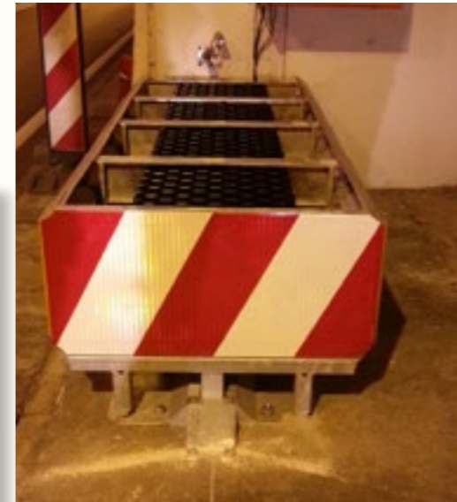
SMA 80P installed in Croatia
